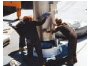
Intermediate level nuclear waste is inserted into an in-ground storage container at the WWMF.
